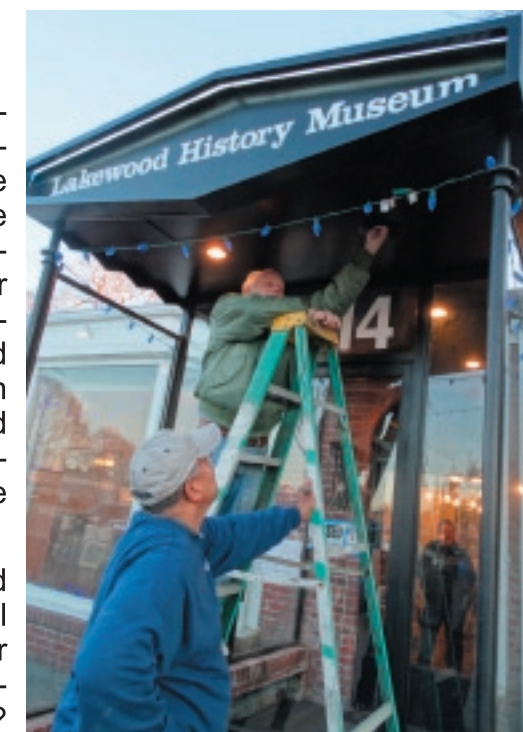
Treasurer Jim Curley steadies ladder while Glen Spieth stretches to reach that last out-of-the-way outlet.
