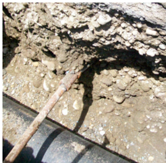
Service line leak
