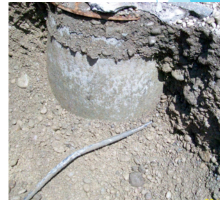
Service line bent
